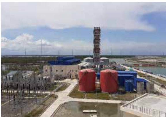
(Mirsarai 150MW Dual Fuel (HFO/Gas) Power Plant)
